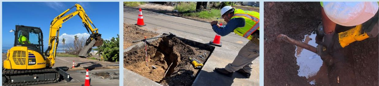
Figure 1: From Left to Right: Crews remove asphalt with a backhoe; An archaeologist inspects the pit; A crew member cuts off a lateral line with a saw.
