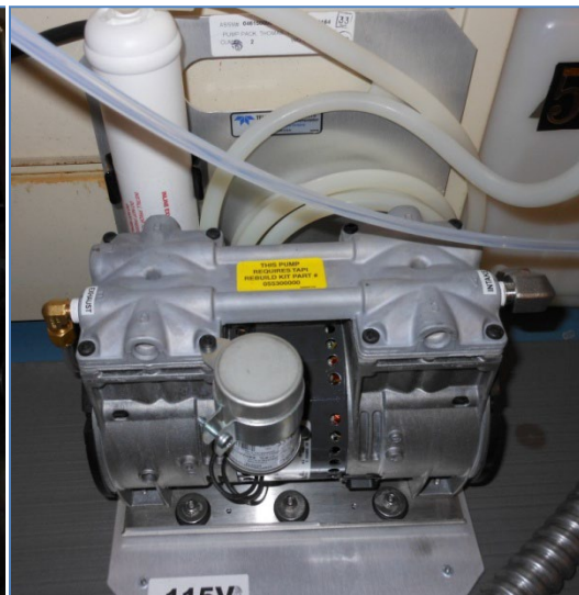
Figure 6. External sample pump
