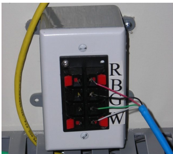
Figure 3. Wall station connecting sensor to data logger
