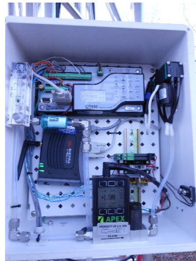
Figure 4. Low Power Enclosure
