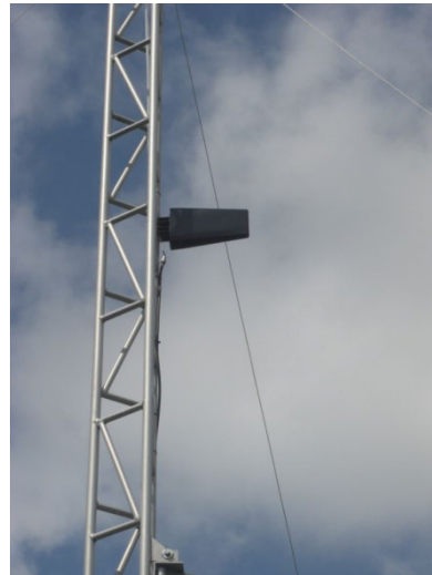
Figure 4. DAS System: Yagi Cellular Antenna Mounted on Folding Tower
