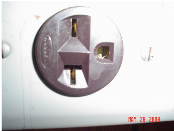
Figure 24. 220VAC Air-Conditioner Power Outlet
