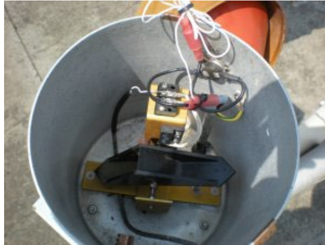
Figure 8. Precipitation Gauge Tipping Mechanism and Wiring.
