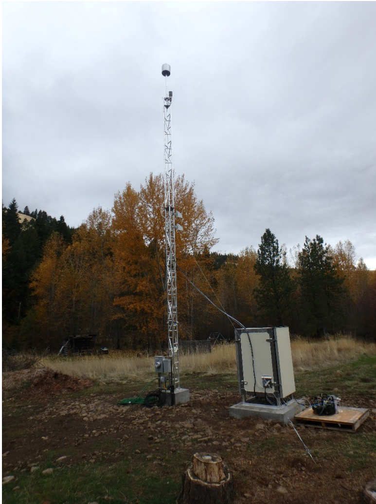
Figure 3. Small Footprint Station with Ozone
