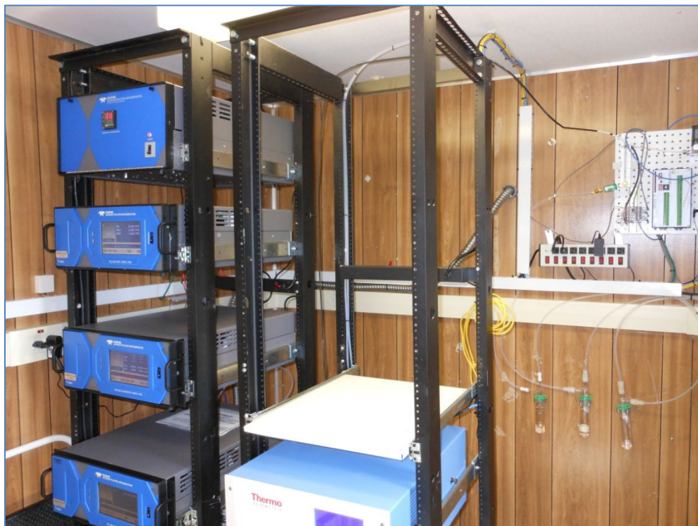
Figure 5. BVL130 Shelter Instrument Rack
