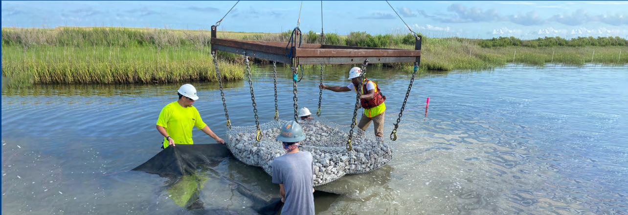
Installing gabion reef units along Sabine National Wildlife Refuge. Credit: The Nature Conservancy
