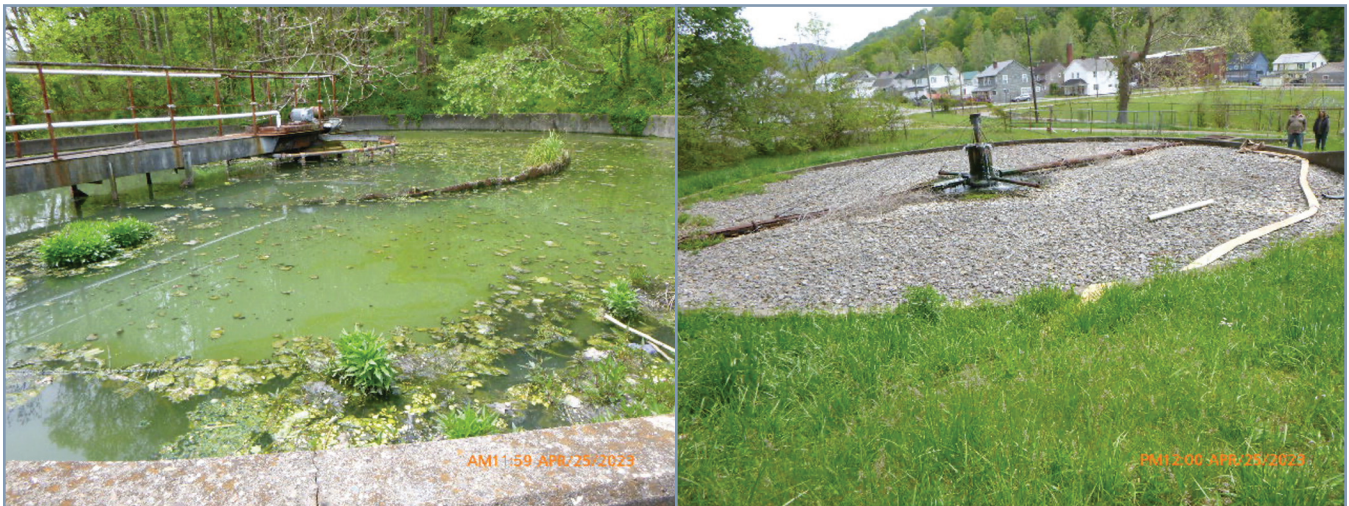
Figure 3. The Lynch WWTP. The clarifier (left), which is not working properly, has excessive vegetation and provides minimal treatment. The trickling filter (right) is also not working properly. Wastewater enters and discharges through the center piping instead of being evenly sprayed through a pipe that slowly rotates.
