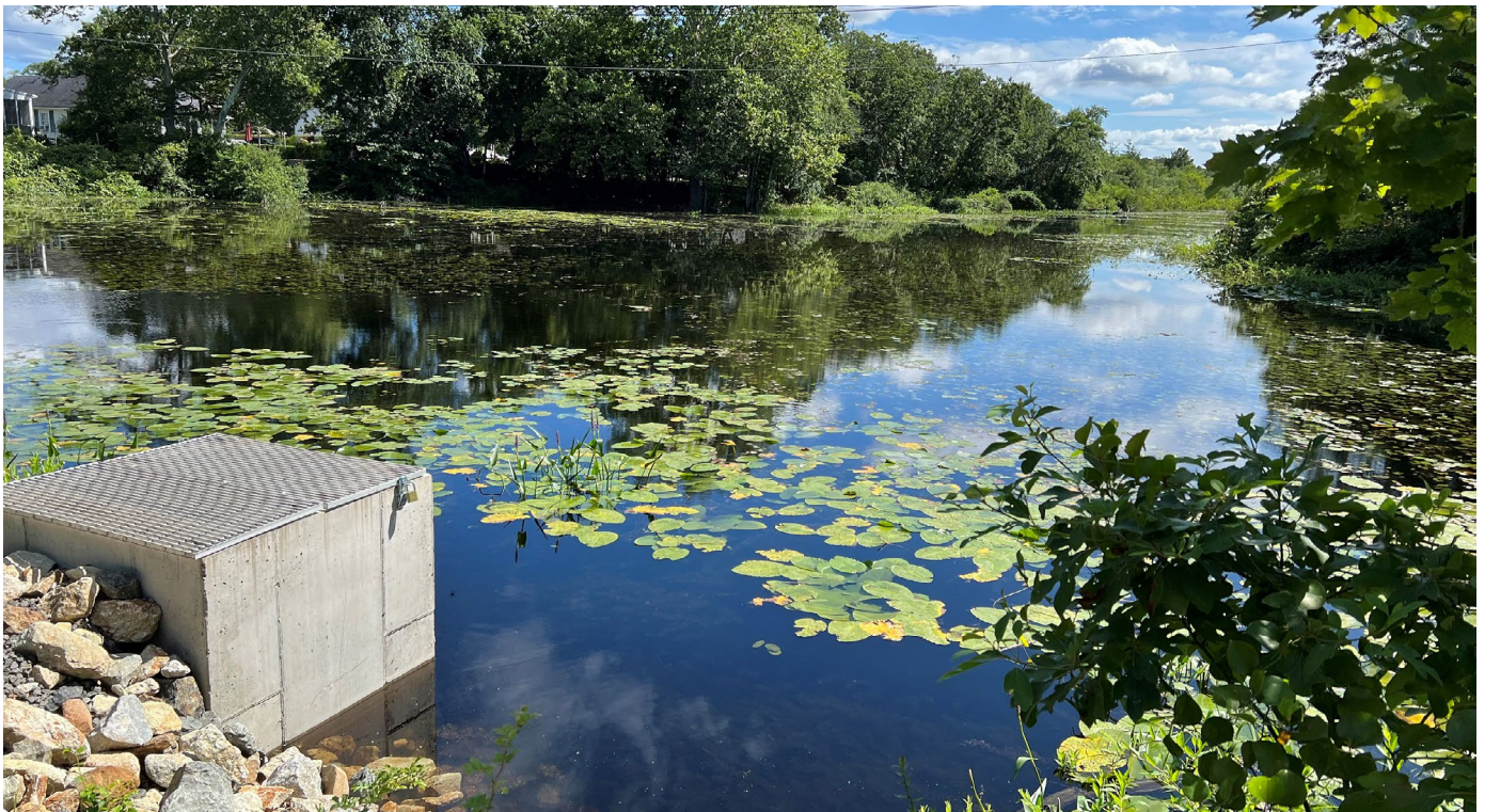
Fish passage structure installed by Peconic Estuary Partnership and its partners. Structures such as this restore critical freshwater spawning and maturation habitat for diadromous fish.
