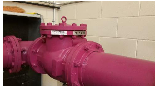
Purple pipes in the City of Meridian, Idaho, which has begun installing water reuse infrastructure with a goal to "recycle and/or reuse 80 percent of the waste stream" by 2030.
