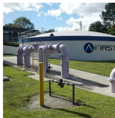
A storage facility with purple pipe distribution in Altamonte Springs, Florida.
