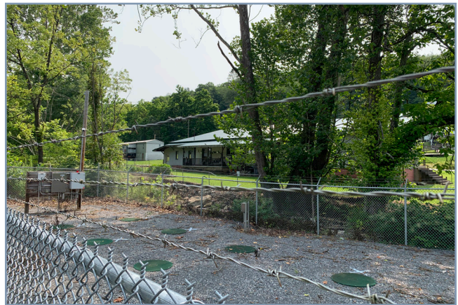
Figure 4. Community septic tanks and lift station in Winona.
