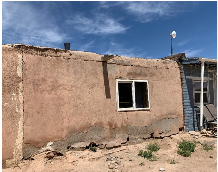
Figure 3. Adobe dwelling affected by water damage.
