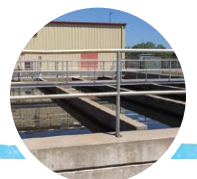
The Heart of the Valley Metropolitan Sewerage District treatment plant (WI) discharges approximately 1.7 MGD treated effluent to a nearby power generating facility for use as cooling water.
