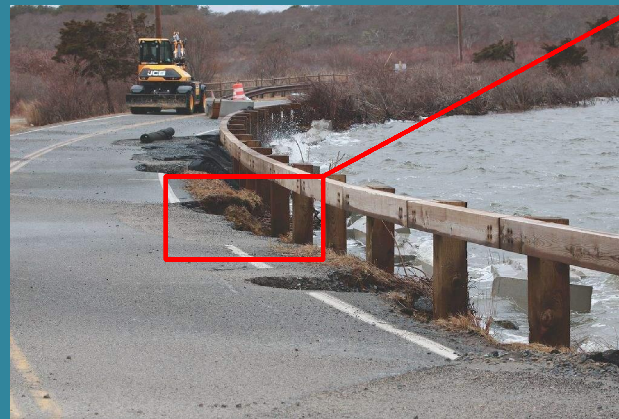
Figure 2. Polpis Road failure from a winter storm in 2018.
