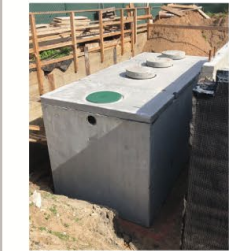
6,000 GALLON UNDERGROUND CONCRETE WATER STORAGE TANK
