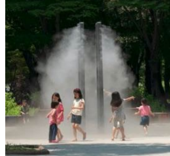
Structure for Water Mist Spray
