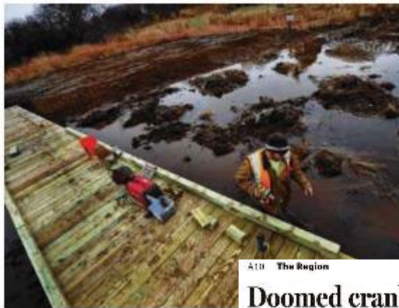
Jeremy Sanders worked on a walkway in Nantucket that is becoming wetland.
