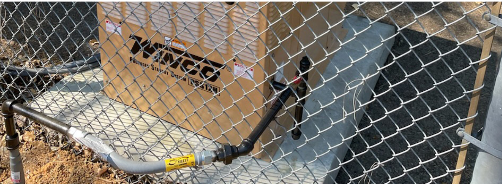
The Cahto Tribe of the Laytonville Rancheria installed this emergency generator for their wastewater system.
