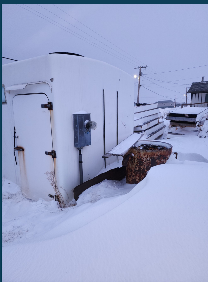
Existing Covenant Lift Station—photo credit CRW.
