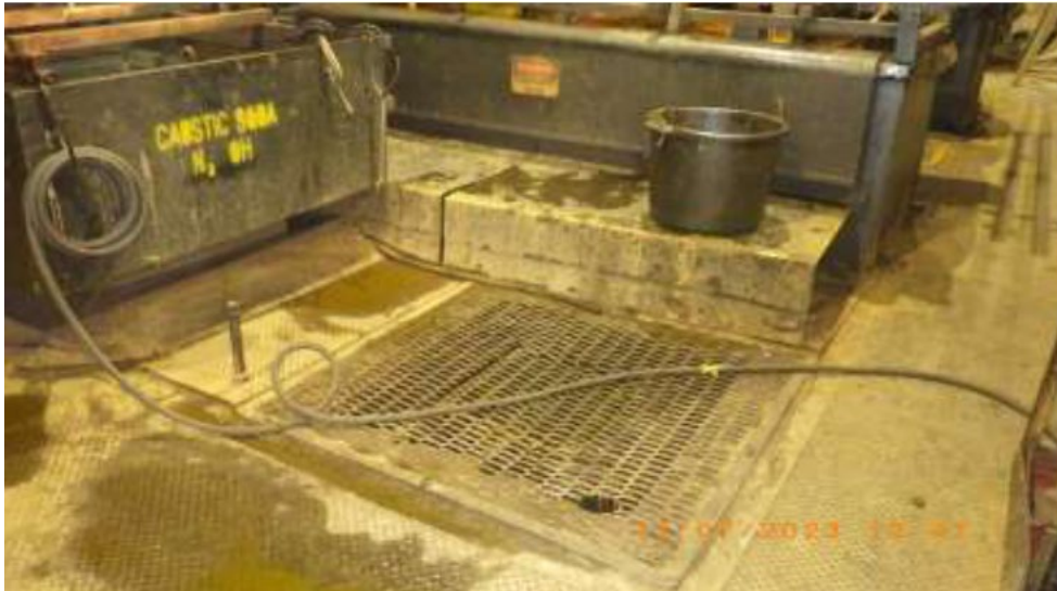
Figure 8 - Plating Rinse Sump
