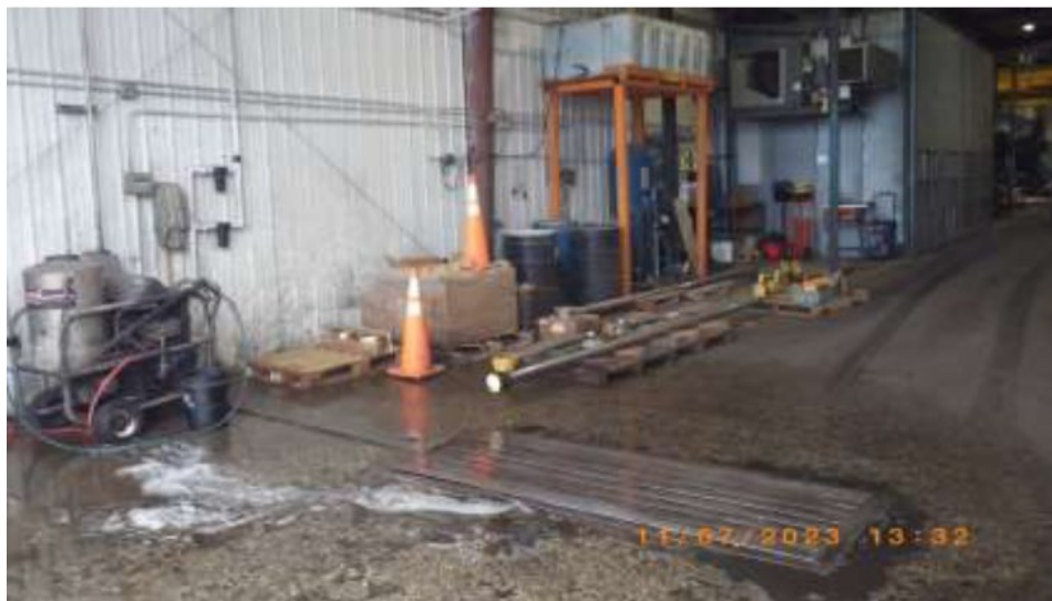
Figure 4 - Steam Cleaning Unit and 150-gallon Wastewater Collection Sump
